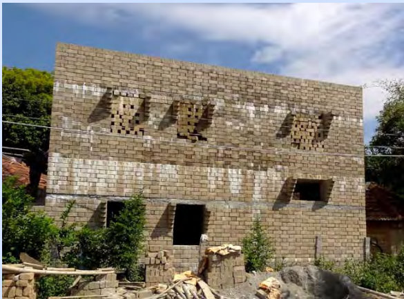
The new OT building coming up donated by FOS [Friends of Sittilingi]
